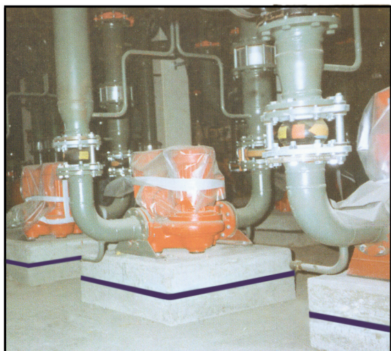
Pump Service Pad Isolation
