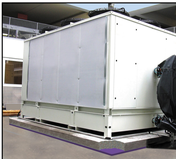
Air Handling Unit Service Pad Isolation
