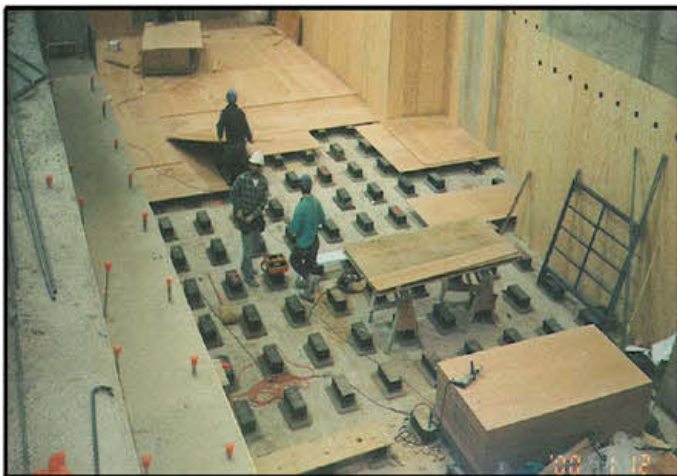
Typical large GK Block foundation under construction. Notice that the workmen are placing the plywood decking that in this case will support the concrete foundation.
